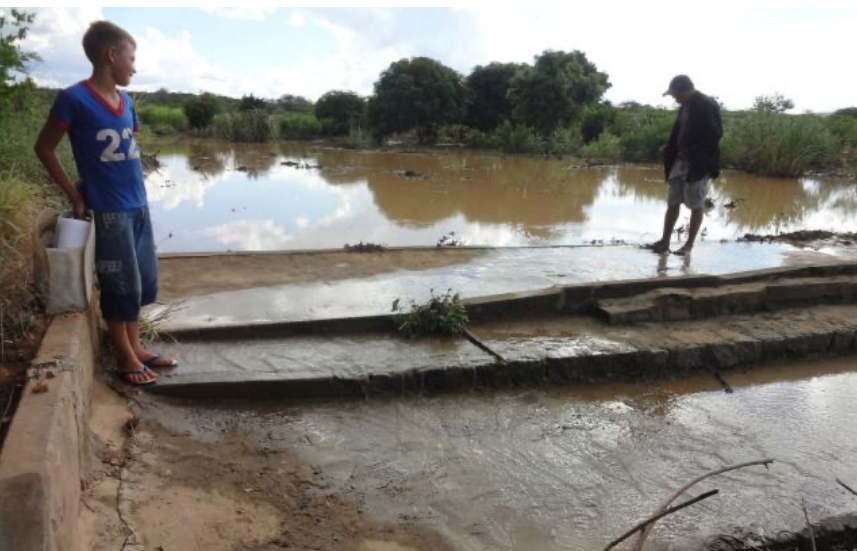
Underground dam after a rain event in Ouricuri, state of Pernambuco (photos: João Mello).
