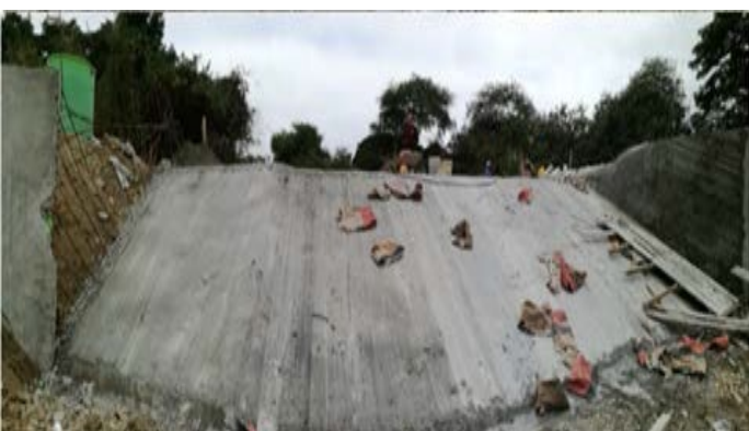
Construction phase of a concrete dike in the Manglaralto river (photo: I. Fajardo).
