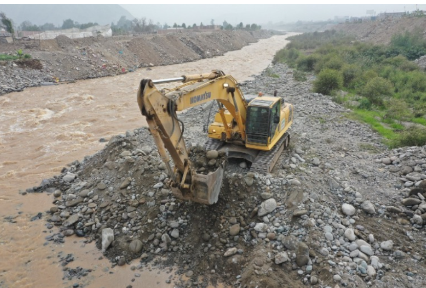
Interventions on the Rimac riverbed to improve infiltration to the aquifer (photo: Revista Perú Construye).
