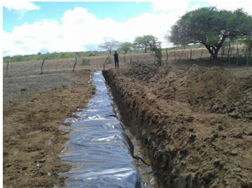
Construction of a sub-surface dam in Campina Grande, state of Paraíba (photo: R. Diniz).
