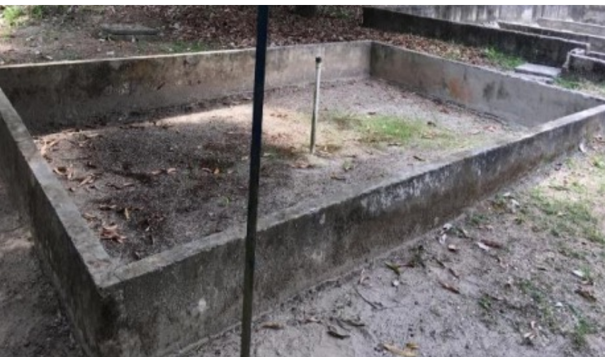
Infiltration trench (photo: José Luis Navarro, 2020).
